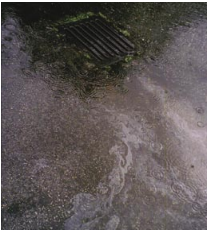
Polluted water flowing into drain
